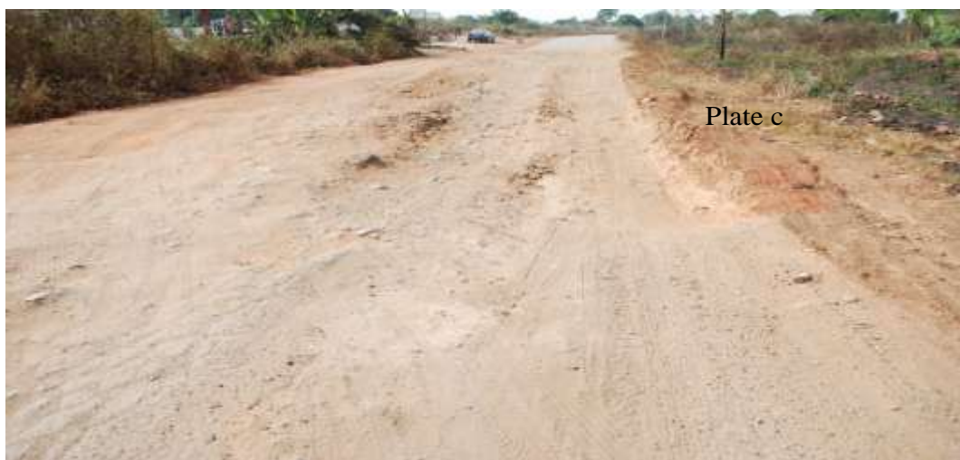
Plate 2. (a) Failed Section at Locality 1; (b) Failed Section at Locality 2; (c) Failed Section at Locality 3.
